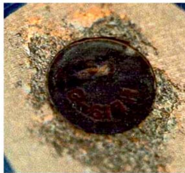
Figure 5. Corrosion around the joint pins
